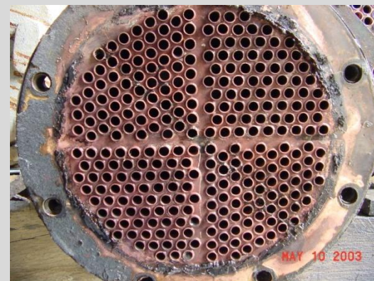
AFTER CLEANING WITH DYNAMIC DESCALER
