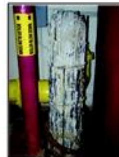
Heater coils before being cleaned with Dynamic Descaler®.
